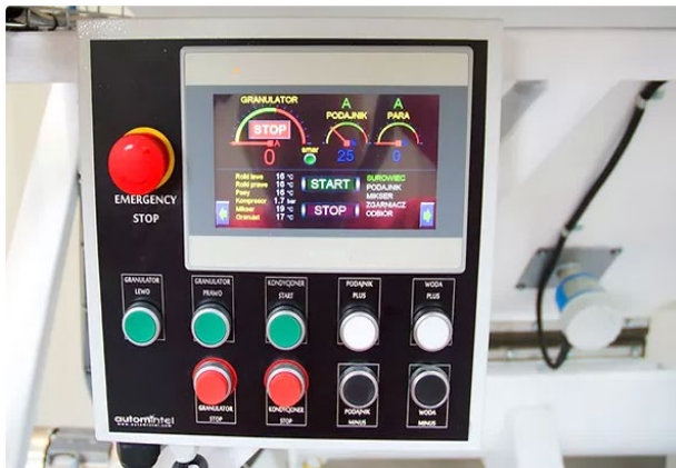
Figure 2 Central Automatic Lubrication System – CALS (Cenei Industrial Park)
