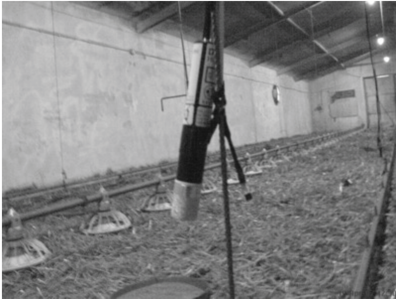
Figure 2 Humidity sensors (left) and temperature sensors (right), at height 0.6 m.
